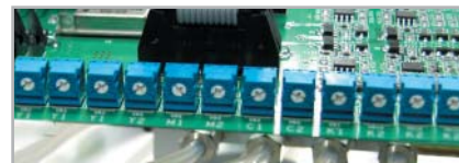
Fire Voltage Control System
